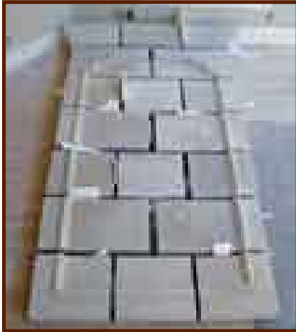
Before starting, layout the stone to dry and verify each piece. Scaffolding may be necessary to work on the upper portions of some mantels.
